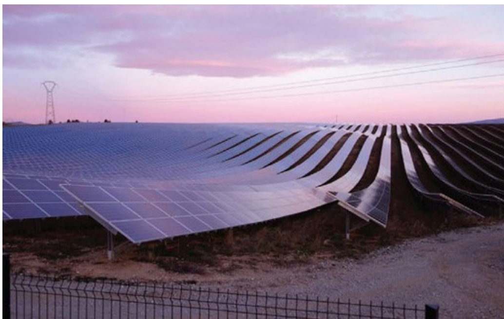
Figure 1. Ground mounted solar array
